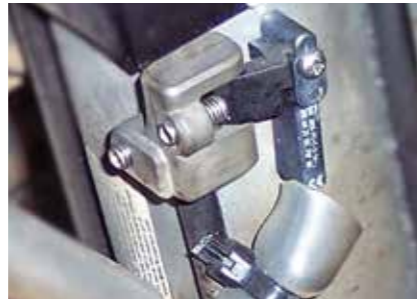
SENSOR CABLE DAMAGE
