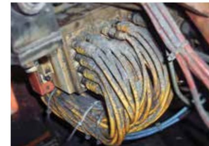
NETWORK I/O BLOCKS DAMAGED
