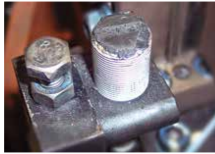
DAMAGE FROM LOADING IMPACT
