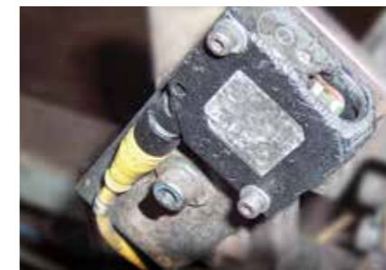
SENSOR DAMAGE BY LOADING IMPACT
